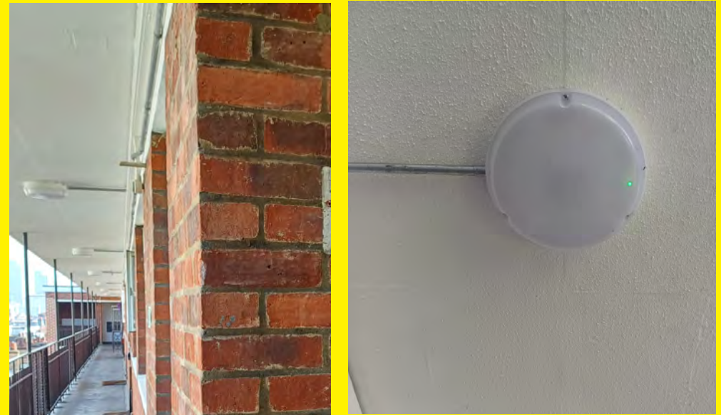
Emergency lighting at Windmill.
