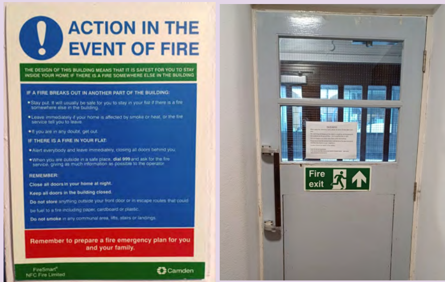
Fire action notice and fire exit sign at Beaconsfield.
