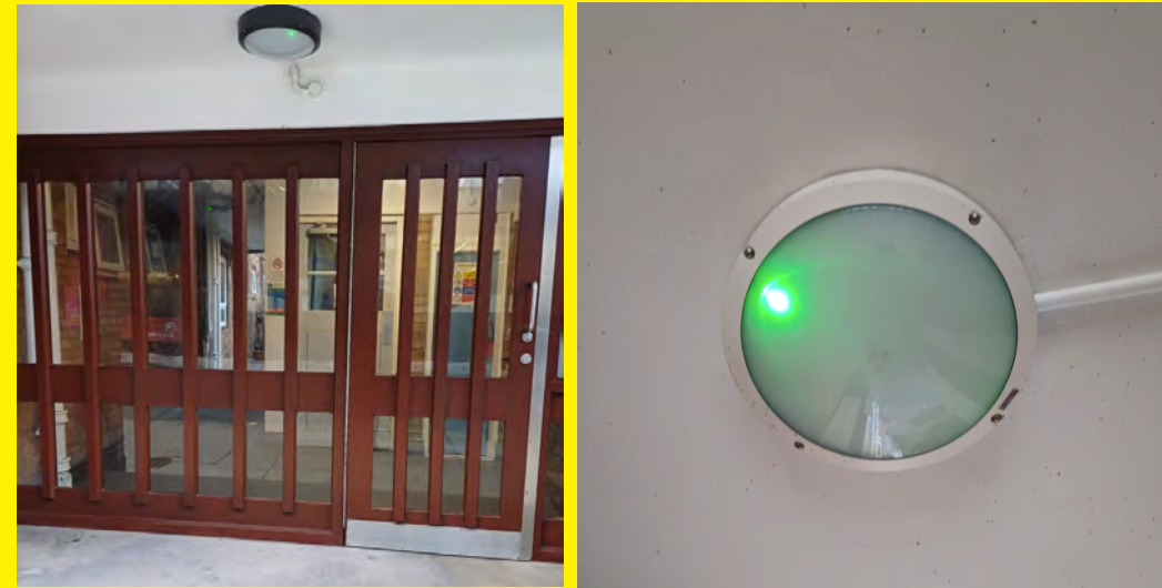
Emergency lighting at Beaconsfield.
