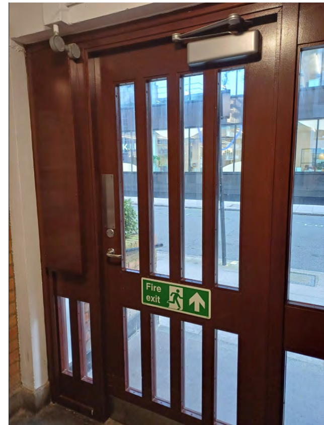
Communal Fire Door at Beaconsfield.
