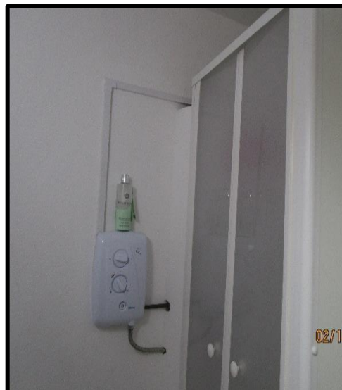
Shower mixer controls located outside of shower cubicle + dangerous wiring
