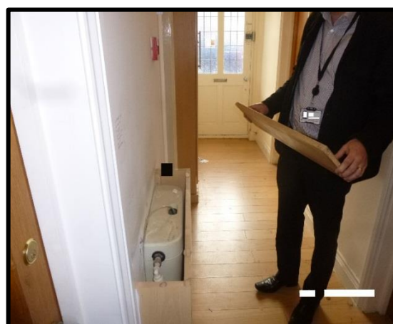
WC cistern for flat located in common parts due to space limitations, resulting in breach of fire separation of wall
