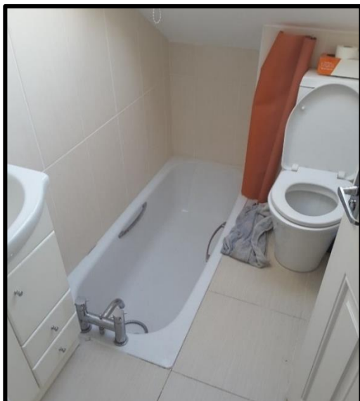
Sunken bath with restricted headroom and smooth floor tiles. Likely to result in trips/falls
