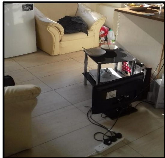
Trailing extension cable across floor and overloading of sockets creating trip and fire hazards
